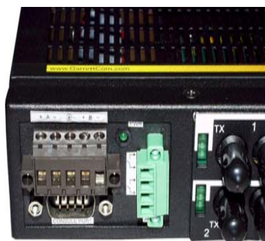
DC terminal block
